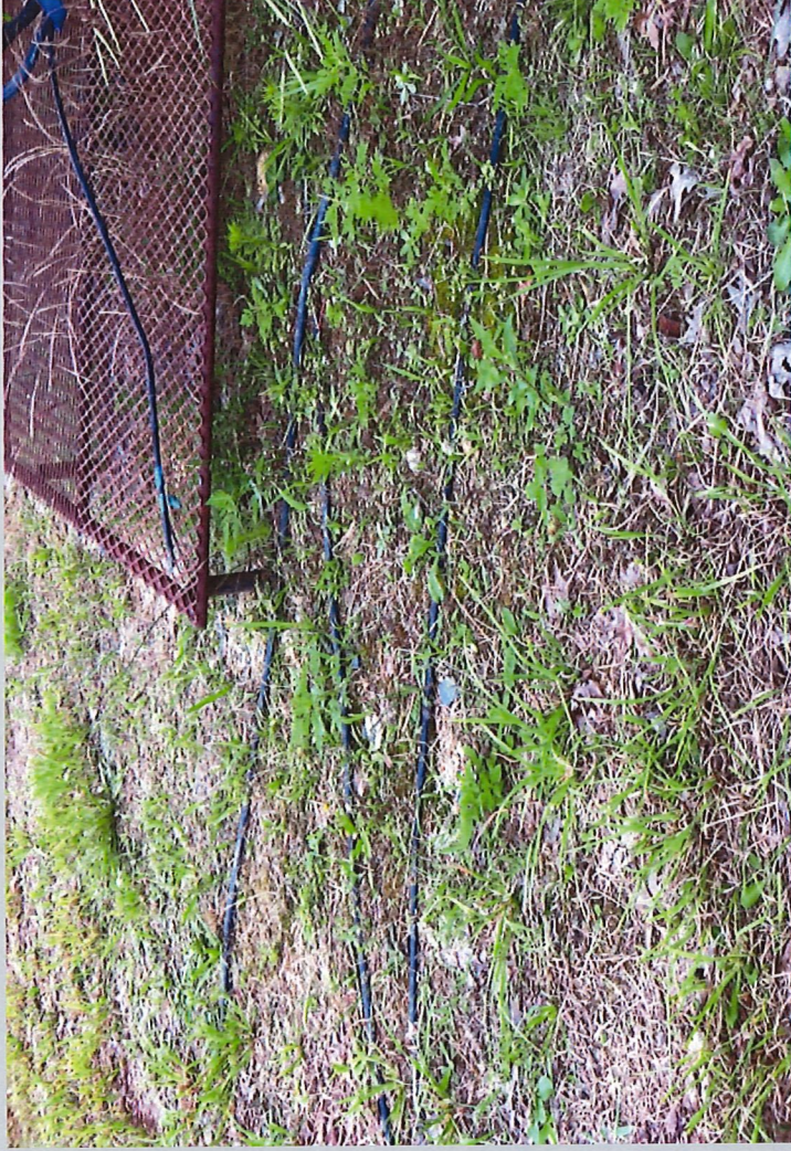
3-phase flexible cables to quarry
